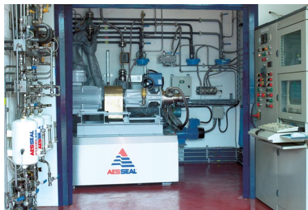
Hot Oil test bay.
